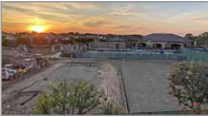
Sport court on the right ready for concrete. Bocce Ball courts on the left.
