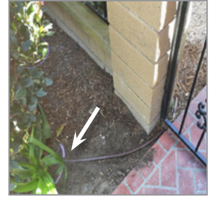
Example of an unauthorized connection to the Association's reclaimed water system.
