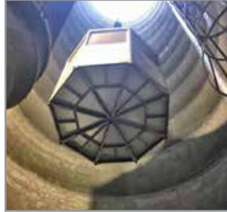
The access point lift for the tunnel project.
